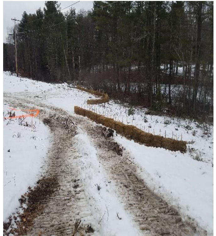
Fig 16: BMPs installed in designated locations along access road to Str. 62. Viewing west. (02-25-20).
