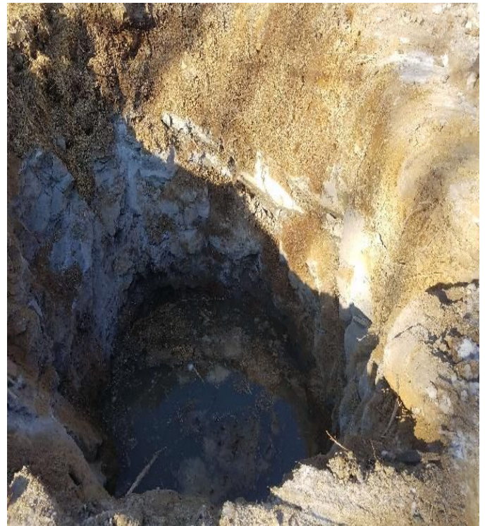
Fig 4: Water in foundation hole at Str. 67. Viewing west. (02-21-20).
