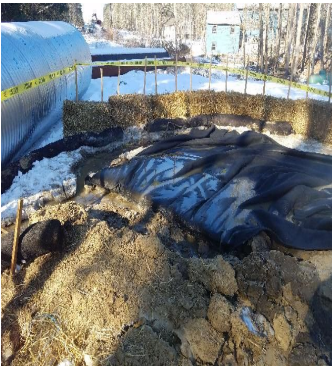
Fig 3: Dewatering basin set up to dewater foundation hole at Str. 67. Viewing west. (02-21-20).
